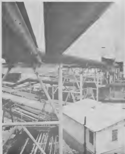
Partial view of 36-inch line (at extreme right) running zigzag on high trestles over pipe banks near Finger Pier No. 3.
